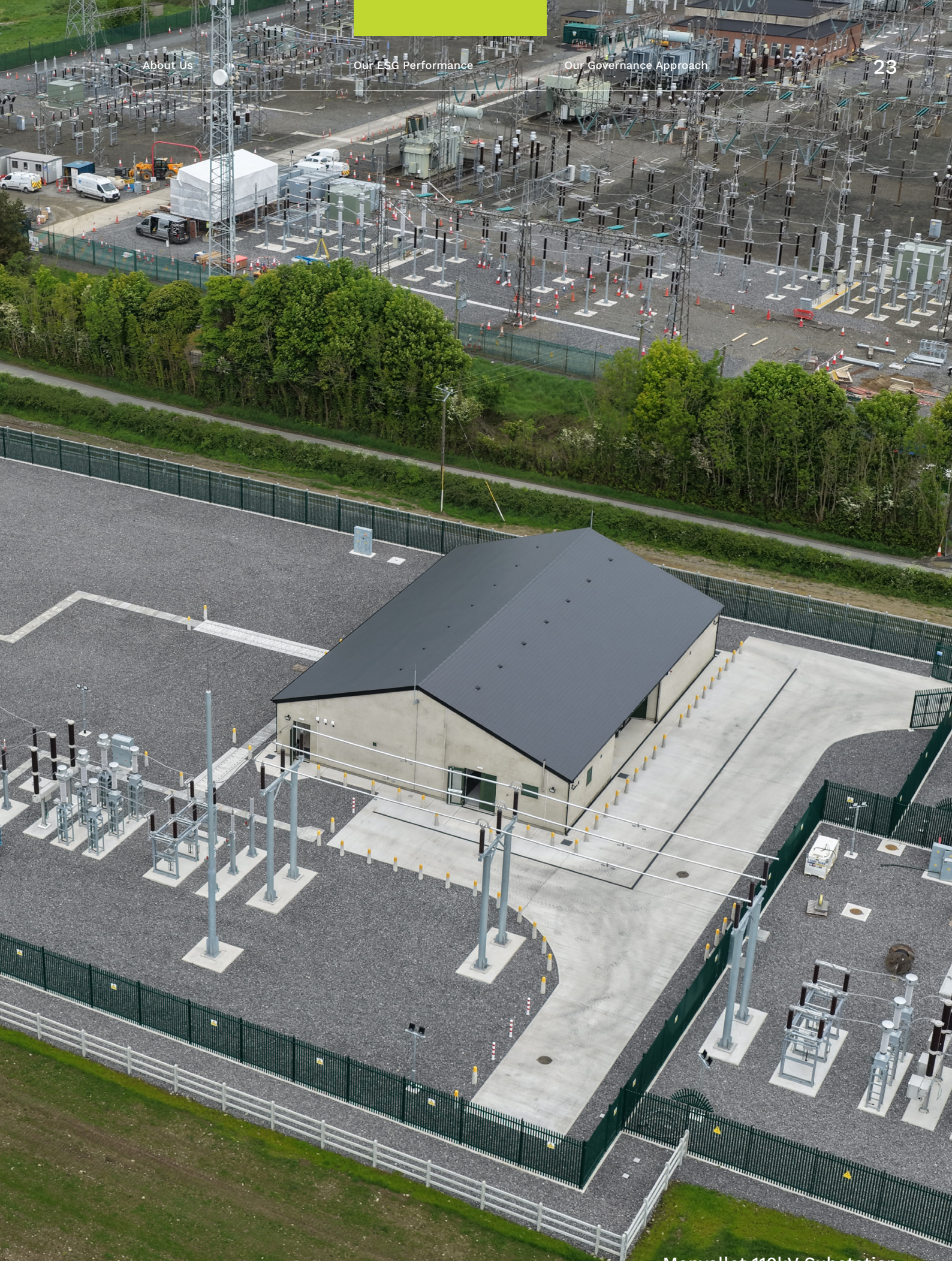
Monvallet 110kV Substation
