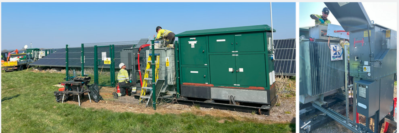
Figure 10: HV improvement works at Brookbarn Apollo Solar site, including the installation of an additional 11kv Circuit Breaker between the site’s two transformer stations
