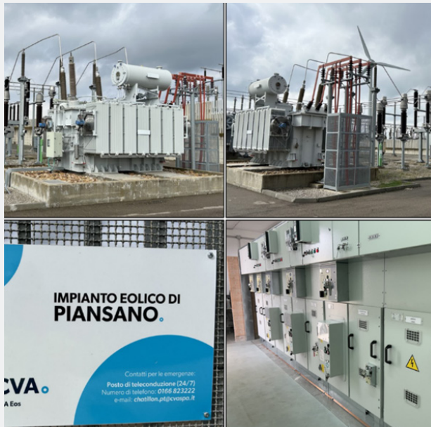
Figure 11: Arlena & Tessennano wind farm’s HV equipment within the Piansano substation in Italy
