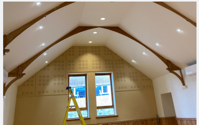
Figure 69: NTR's community benefit fund supported the installation of a new ceiling at Preston Village Hall, Scotland.
