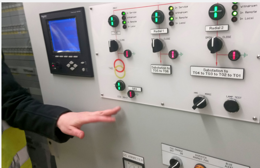
Figure 89: Wind Turbine Switchgear Control Panel
