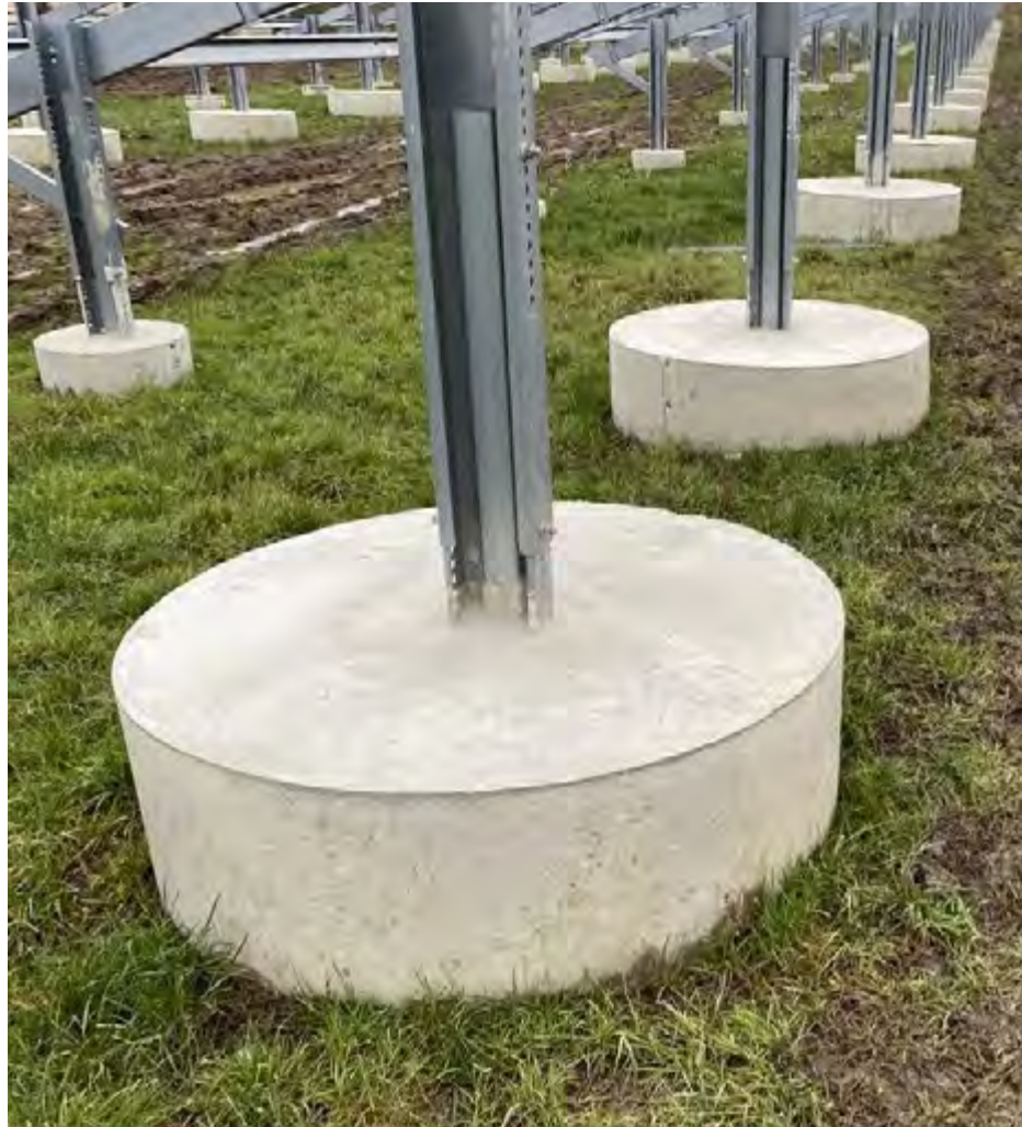
Figure 68: A row of ballast foundations. Note the foundations at the high end of the mounting structure are larger than the ballast at the lower end of the structure as the high end takes the highest amount of wind force.
