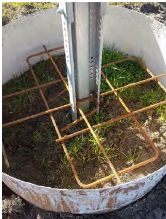
Figure 67: A shallow pile together with reinforced steel linking the ballast foundation to the pile. A mould surrounds the pile which is used to hold the concrete ballast until set.
