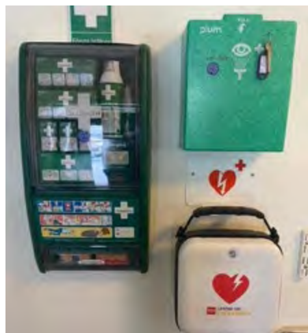
Figure 32: First aid station in the site office at Trattberget, Sweden
